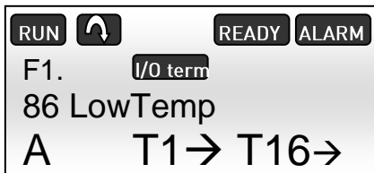
Figure 7.1-3, Low temperature alarm on the NXP panel
